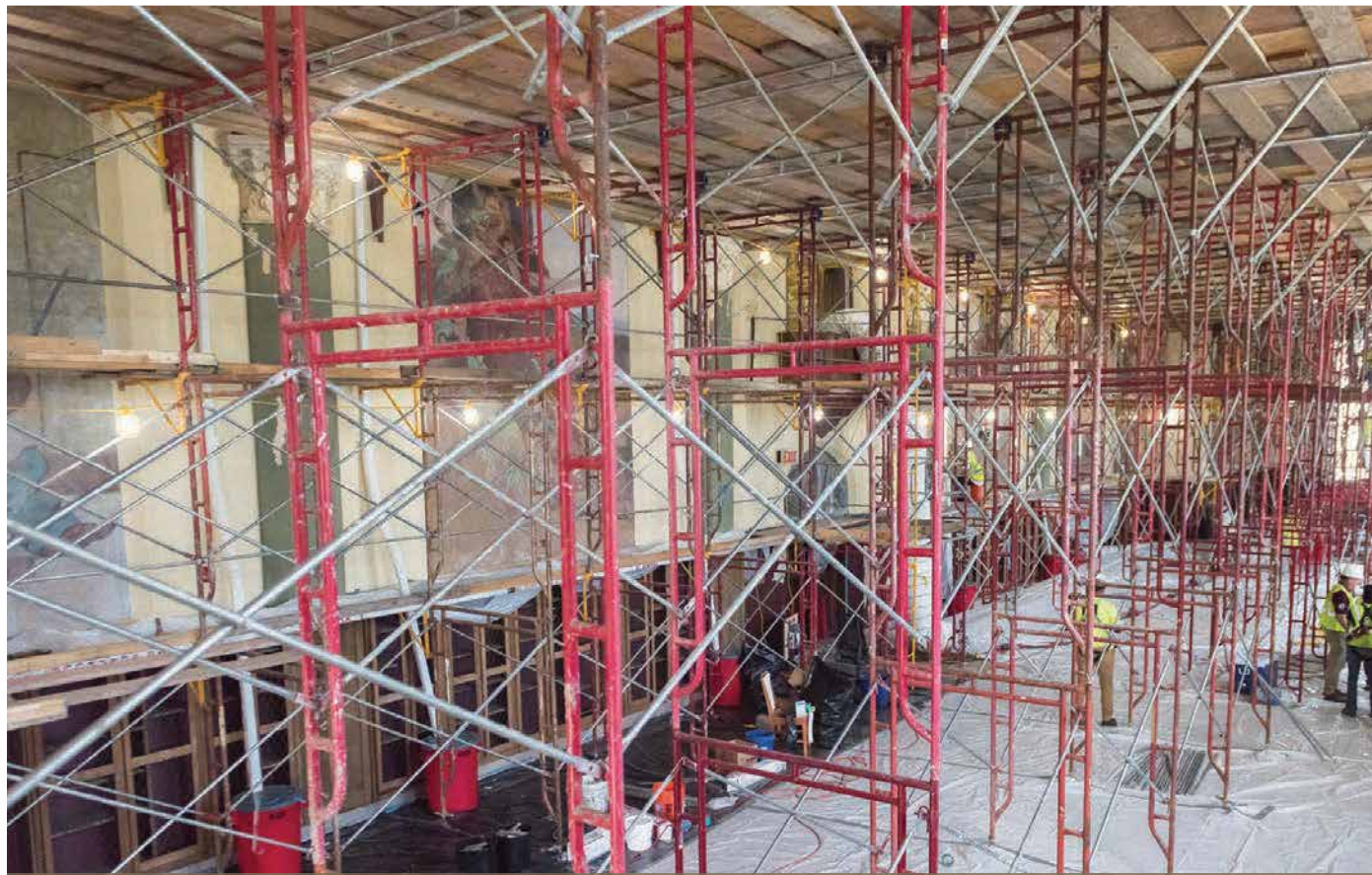
The walls in the Great Room absorbed a lot of water, which put the murals in jeopardy. Conservationists used the scaffolding to monitor the plaster, clean the murals and otherwise ensure their safety until they can be fully restored.
