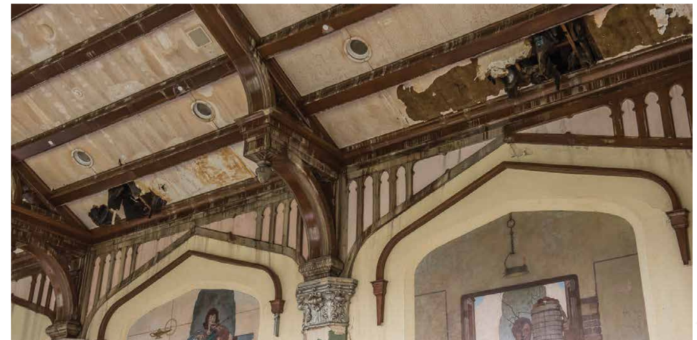
The fire burned through the south side of the Great Room roof in two separate places. While the murals below suffered extensive water damage, every effort will be made to save them.
