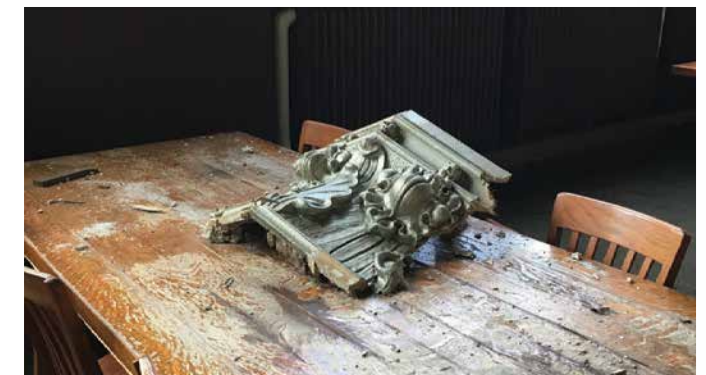
Portions of plasterwork were damaged by water and fell from the walls, like this decorative capital.
