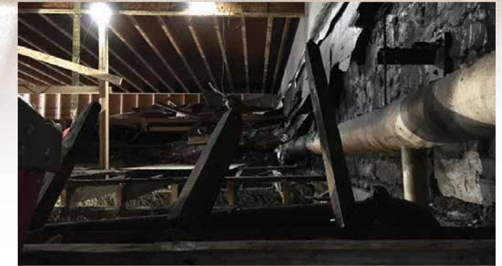
Portions of Farrell Library's roof, attic and ceiling were destroyed. The hole was covered by a temporary roof (at top); charred plaster, debris and beams remained.
