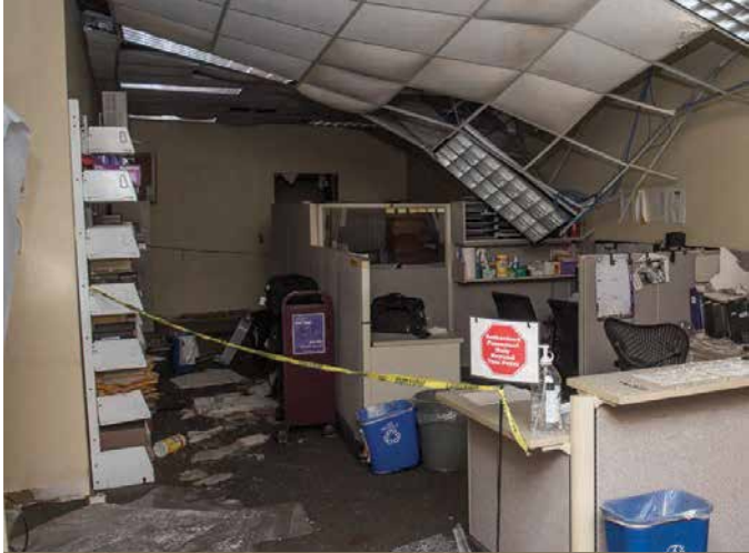
A collapsing drop ceiling drapes over the equipment check out desk. Water cascaded from the Great Room into information technology offices on the second floor.
